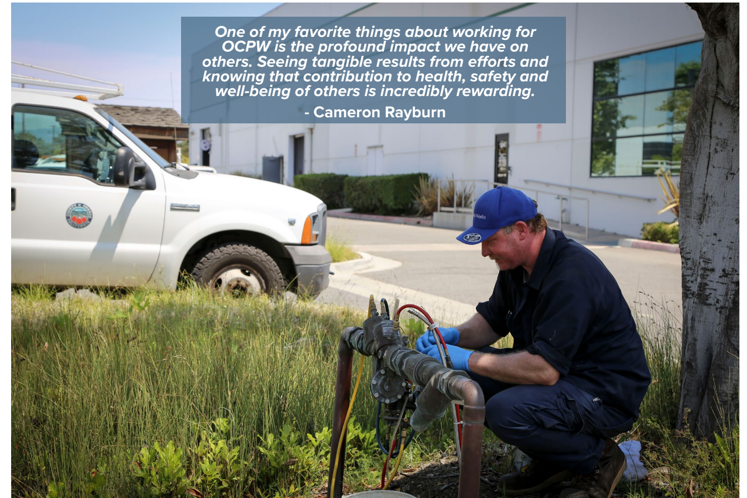
Cameron does a routine maintenance check on a backflow system valve at the Glassell Campus.
