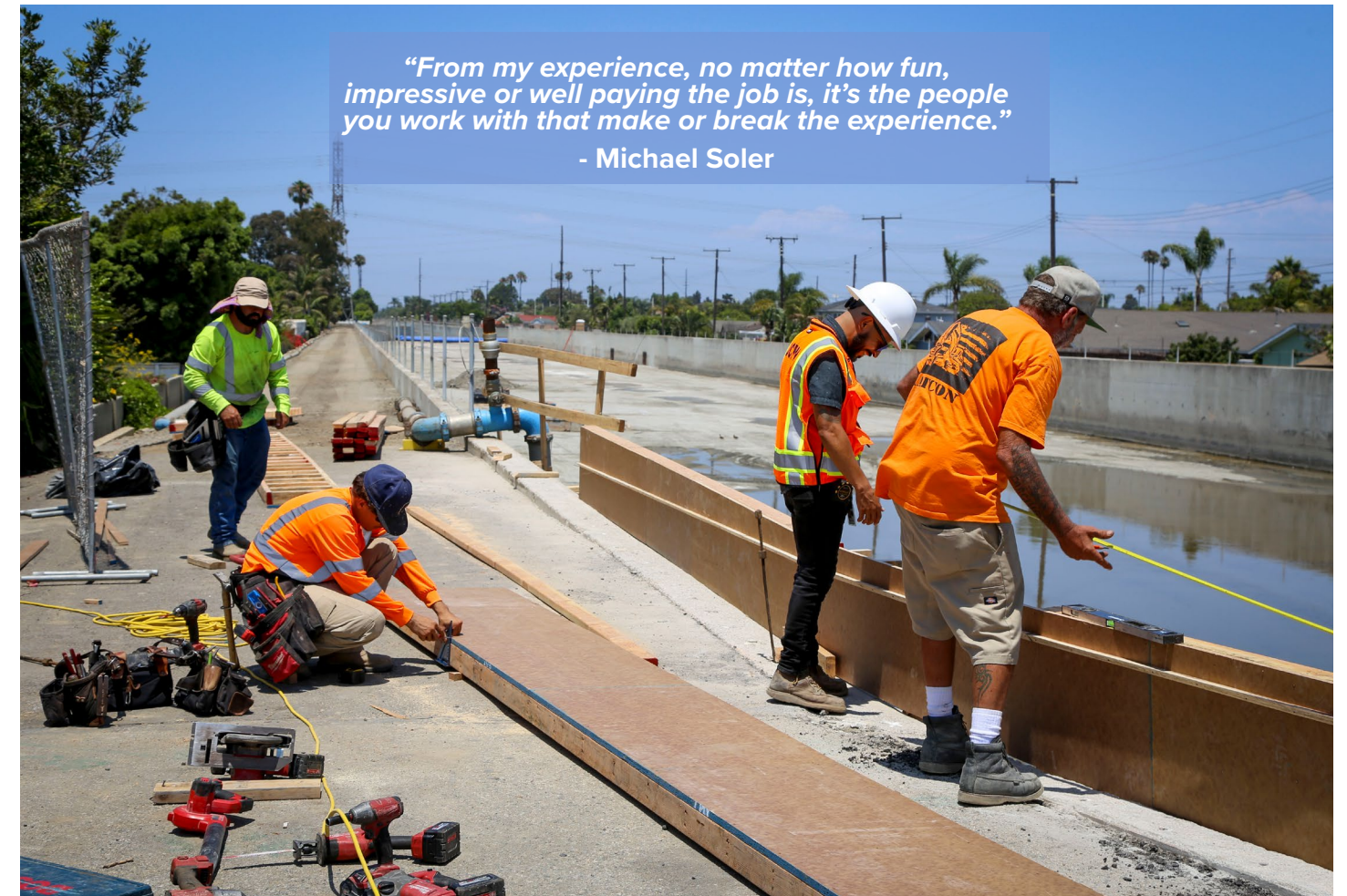
Michael and his crew are constructing channel wall improvements along the Talbert channel in accordance with FEMA regulations.
