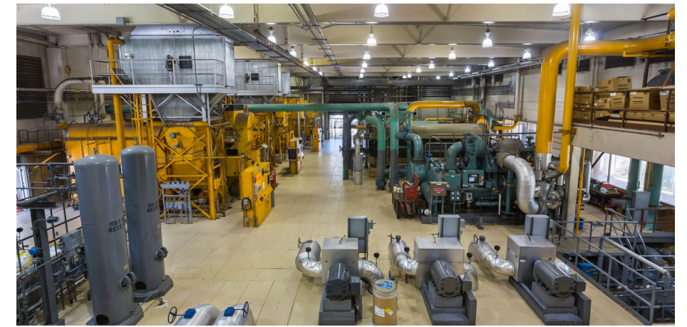
Inside the Central Utility Facility in Santa Ana
